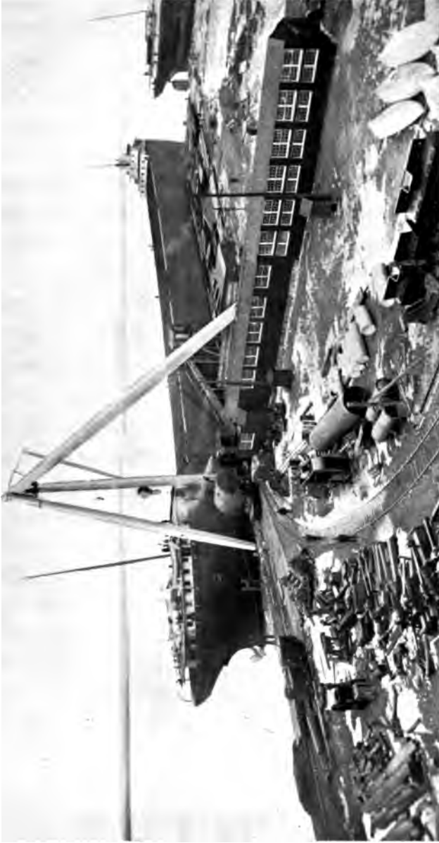
The "Thomas F. Cole," 11,200 Tons, Being Fitted with Engines and Boilers after her Launching.
